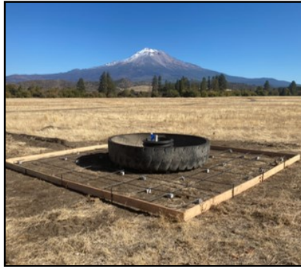
Photo: Construction of off-channel stockwater trough with healthy Parks Creek riparian corridor and Mt. Shasta in background.
