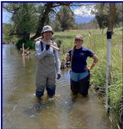
Jose and Mallory installing a stilling well to track flows and measure project efficacy in the Upper Shasta River.
